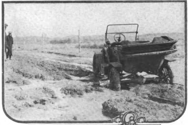
Lack of proper side-ditches is emphasized.
